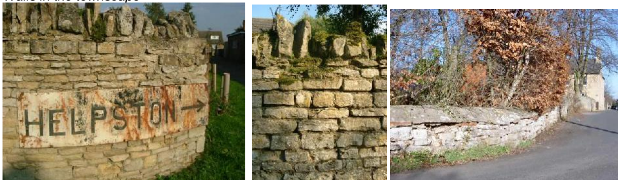
Wall in poor repair
